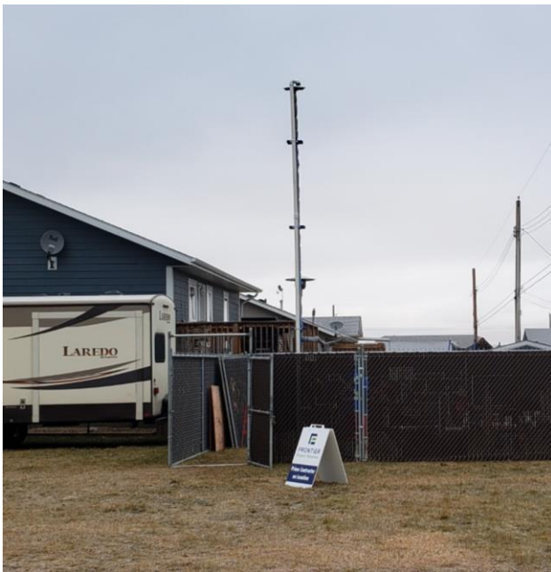
New dual vent stack within the fenced enclosure
